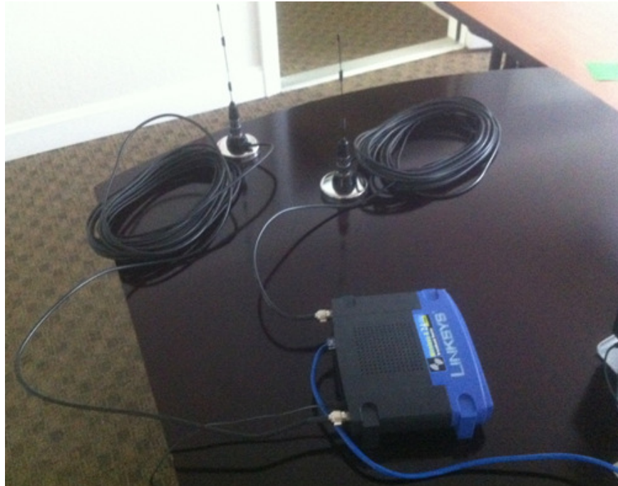
Figure 56 Antenna connected to Router
