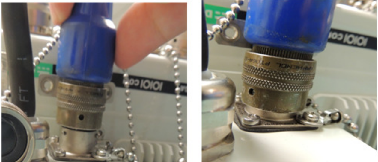
Figure 45 Power cable connected to the Azonix
