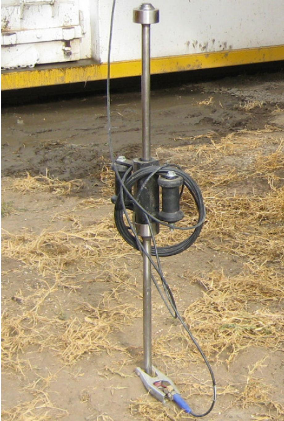
Figure 96 Ground stake 02JIGS008 driven 3 feet into the Ground Cable 22CABL0058 and Clamp 02X-EM0088 “on to the Ground Stake
